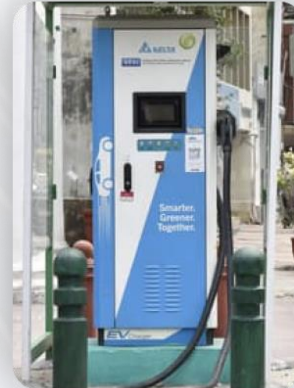
Poor charging infrastructure
